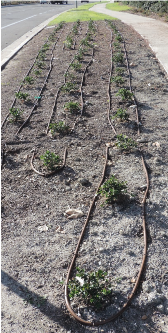
Turf replacement project. This in-line drip system is not installed correctly. The emitters are too close to the plants. In-line drip should be engineered to wet all the soil through gravitational and capillary action. You need to match the soil type and the plant's root depth/water needs to the emitter flow rate and hose spacing. The goal is to provide 1 - 1.5 (up to 2) inches of precipitation with each irrigation to all the soil, with no soggy spots or dry spots.
