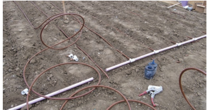
In-line drip installation. If engineered correctly, all the soil will be uniformly irrigated because the designer chose the emitter flow rate and the hose spacing based on the soil type and the water needs of the planting.
